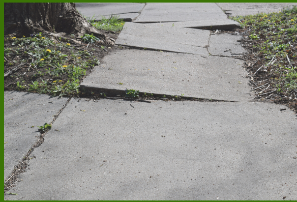
TREE ROOTS & UNEVEN SURFACE
